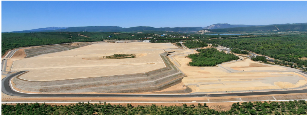
Figure 3-2 – The ITER platform in Cadarache, where construction will begin in 2010 on buildings and facilities
