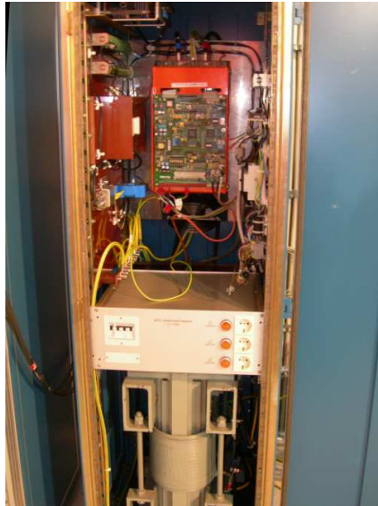
(a) Power supply cubicle
