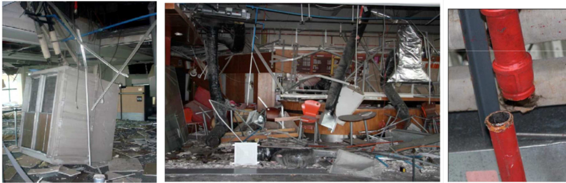
Figure 1.45 damages to utility system components at Santiago Airport (Miranda et al. 2012)
