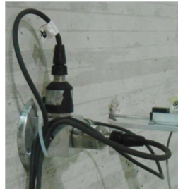
Figure 2.16 Example of acceleration sensors installed on the wall surface opposite to that of anchor installation
