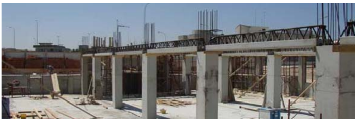
Fig. 1.4: Leone's composite steel truss and concrete beams with the inferior concrete base (Italy)
