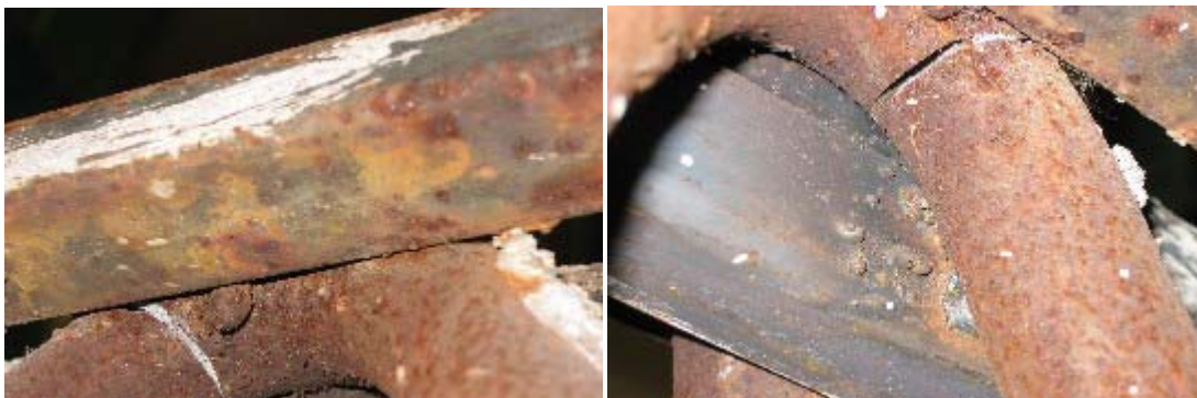
Fig. 4.74: Pictures of the diagonal bar fractures: beam 1 (a), beam 2 (b)
