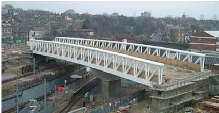
Fig. 1.2: Pedestrian composite steel and concrete truss bridge of Arsenal's Emirates Stadium (United Kingdom)
