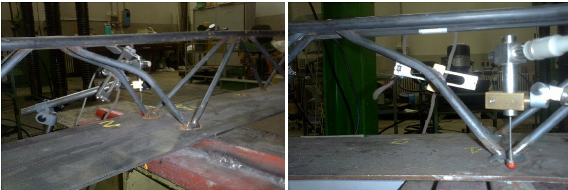
Fig. 4.13: Pictures of the trusses 2 after the collapse
