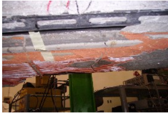
Fig. 4.39: Picture of the lower clay tile in the beam 101 mid-span close to the collapse
