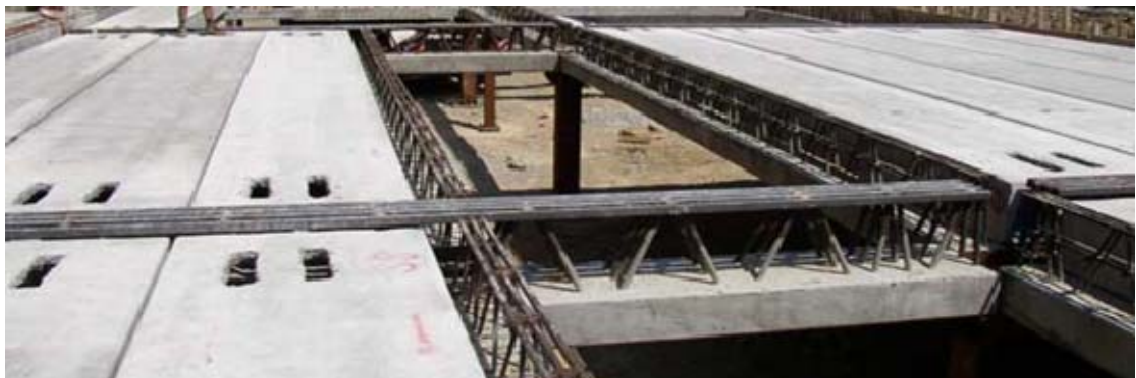
Fig. 1.6: Pictures of the use of CSTC beams with first phase self bearing slab (Italy)
