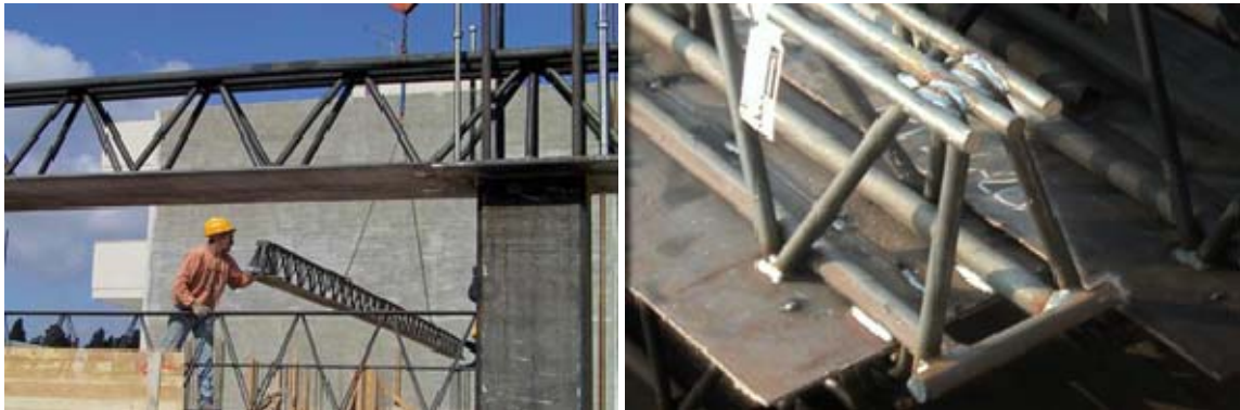
Fig. 1.3: Leone's original composite steel truss and concrete beams with the inferior steel plate (Italy)
