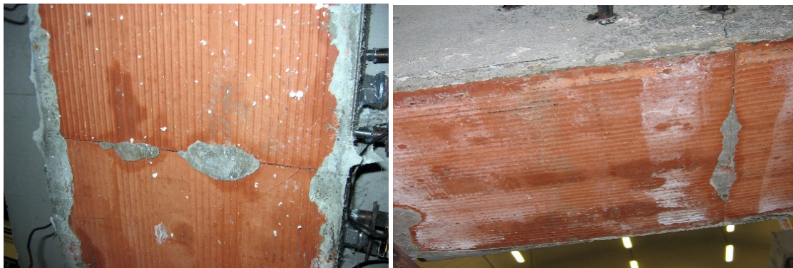
Fig. 4.51: Pictures of the lower clay tile in the beam 103 close to the collapse
