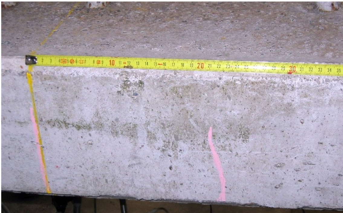
Fig. 4.69: Picture of the crack distance
