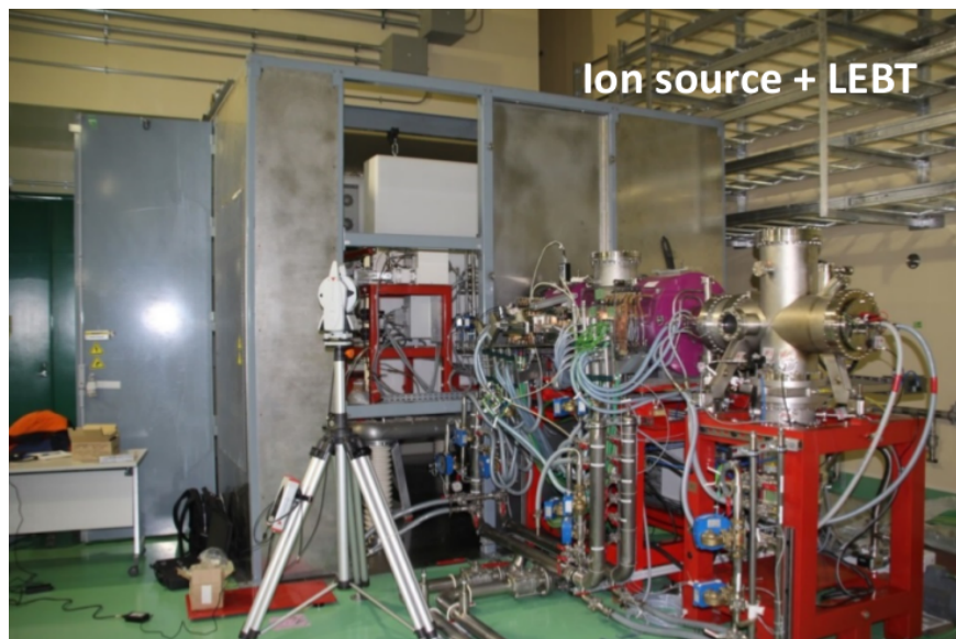
Fig. 3.3 Photo of the LIPAc injector installed at Rokkasho
