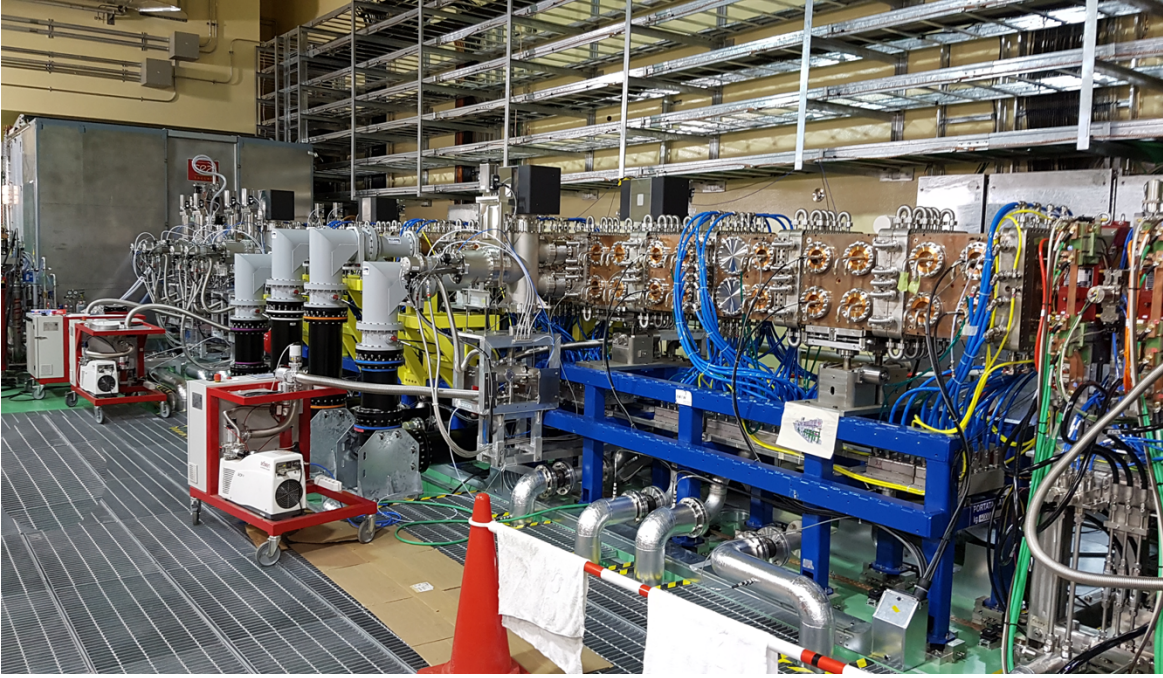
Fig. 3.18 RFQ installed at LIPAc facility
