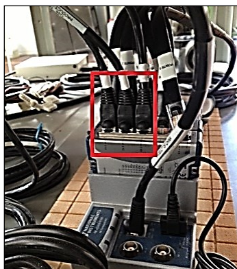
Figure 23: Cable connections to the NI-9237 for “Mototiremeter”
