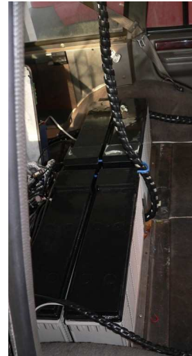
(b) UPS batteries detail
