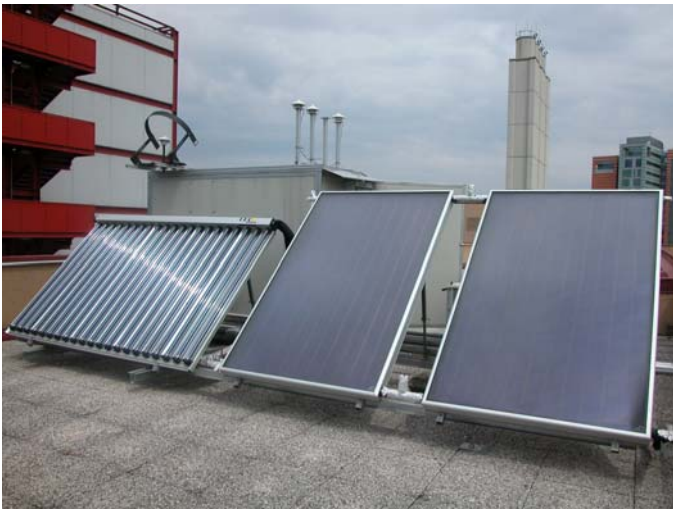
Figure 2. Collectors installed in the test apparatus.
