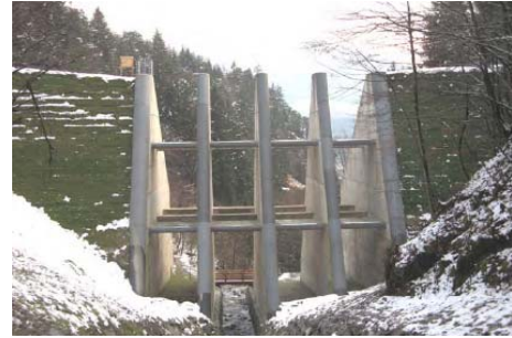
Fig. 4.50 – Catching dams: a) arresting walls; b) catching dams; c) breaking dams [ http://cagem.bayindirlik.gov.tr ; McClung & Schaerer, 1996; http://cemadoc.cemagref.fr ; Pittracher, 2008].
