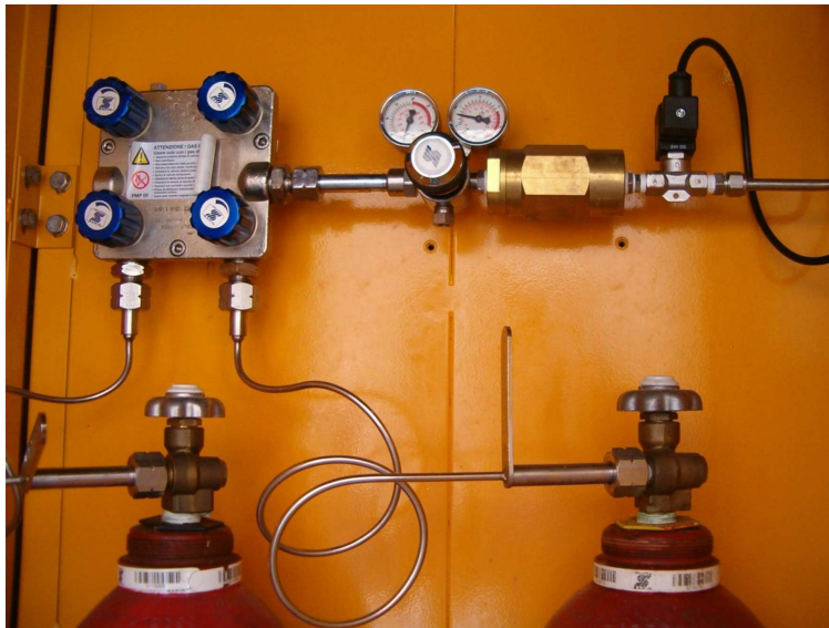
Figure J.10. High and medium pressure hydrogen fittings.
