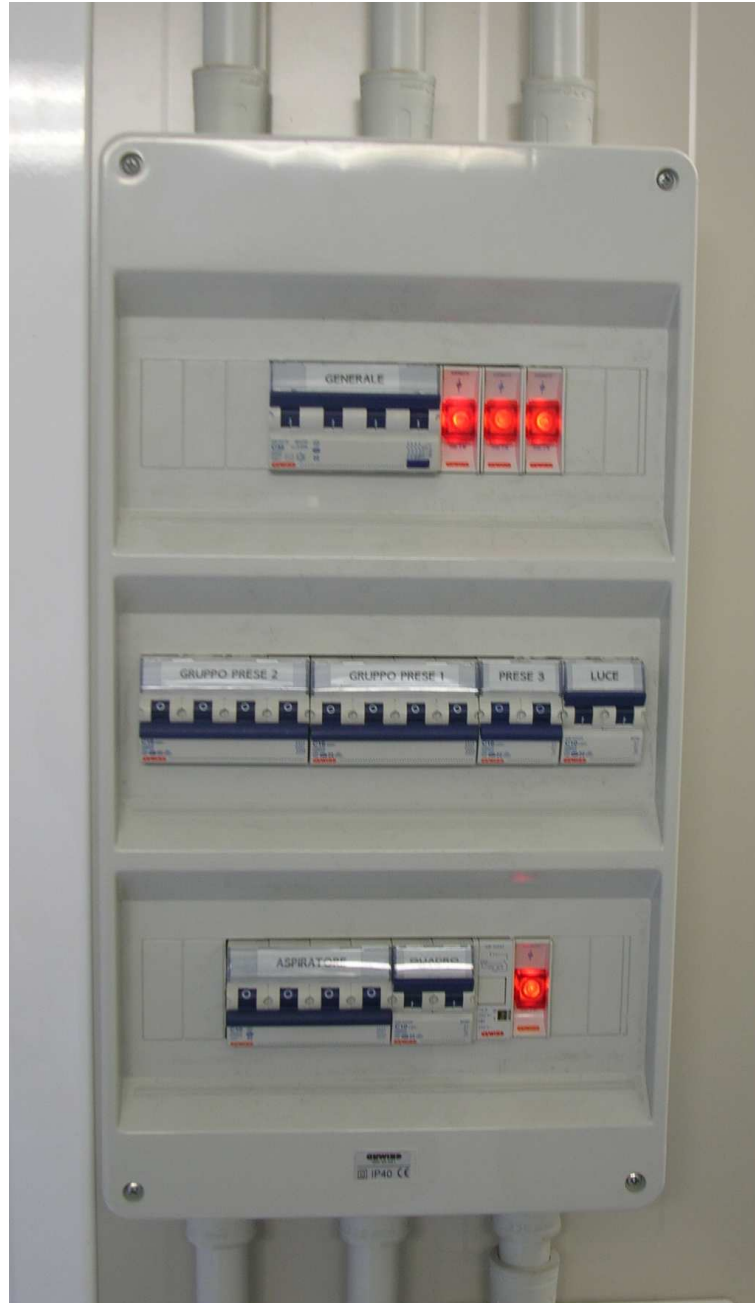
Figure J.6. Main electric panel.
