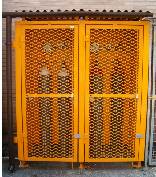
Figure J.11. Oxygen and hydrogen cylinder cabinets. The cylinder in use must have the yellow label “ Bombola in uso ” (“Cylinder in use”). The new cylinder must have the yellow label “ Bombola carica ” (“Full cylinder”). Empty cylinders must have the red label “ Bombola scarica ” (“Empty cylinder”).
