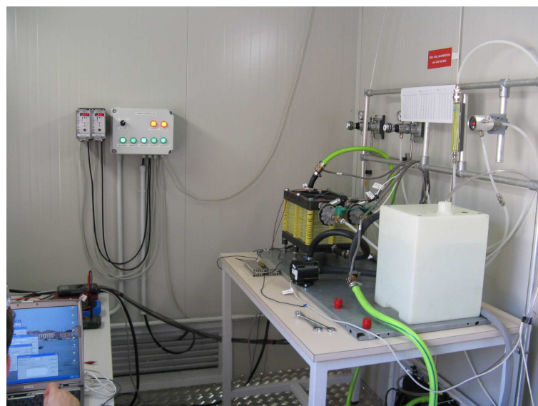
Figure 5.4. The fuel cell stack after installation. The inlet valves are connected to the hydrogen and oxygen systems with two flowmeters in series. The outlet valves are connected to two pipes that carry the gasses outside. The radiator has been oversized and put under the table. A 100 k \Omega resistance is always connected in parallel to the stack, in order to avoid to keep it in an open circuit state.
