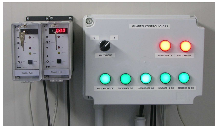
Figure J.5. The gas safety system. On the left are the hydrogen and oxygen concentration measurement units. On the right is the panel with all the safety controls (green lights). The gas solenoid valves (red lights) are open only if all the safety controls are passed.
