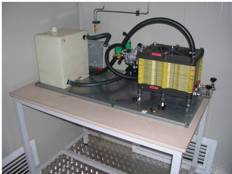
Figure 5.2. The fuel cell stack with the coolant tank, pump and radiator. On the right of the stack, there are the two outlet valves.
