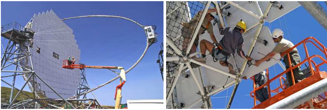
Figure 4.34: Two phases of the installation of the mirrors in the telescope. The mirror is taken to the reflector front via a cherry-picker (left) and the mirror is fixed by operators to pads mounted on the telescope structure.
