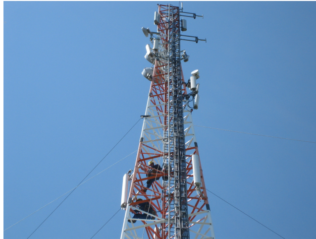
Fig. 1.6 Example of base station antennae.
