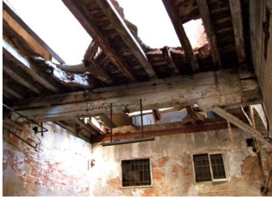
Fig. 4.4.17: view of the beam before the interventions to provide safety conditions of the wooden floor
