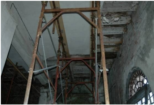
Fig. 4.4.26: Collapse of the false ceiling next to the masonry
