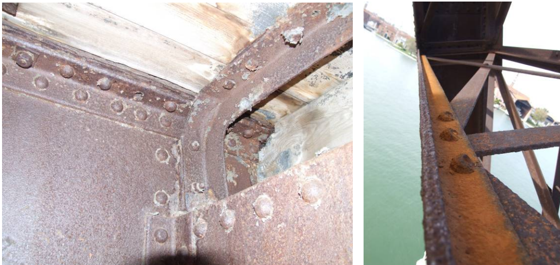
Fig. 5.8.14: Details of missing or degraded rivets
