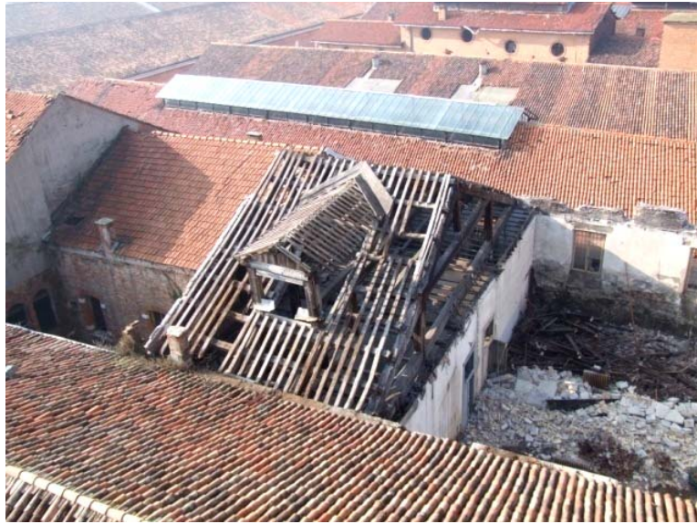
Fig. 4.3.25: View of the partially collapsed wooden roof
