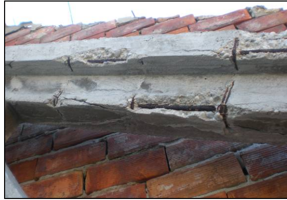
Fig. 4.4.113: Detail of a lack in a strut
