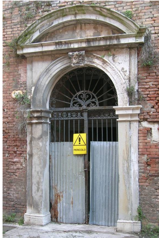
Fig. 4.2.6: Entrance portal of the northern “Sale d’Armi” on the “Stradal Campagna”
