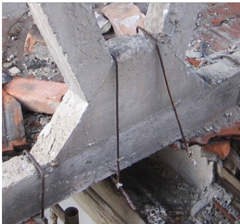
Fig. 4.4.115: Detail of the connection hook between false ceiling and the tie beam
