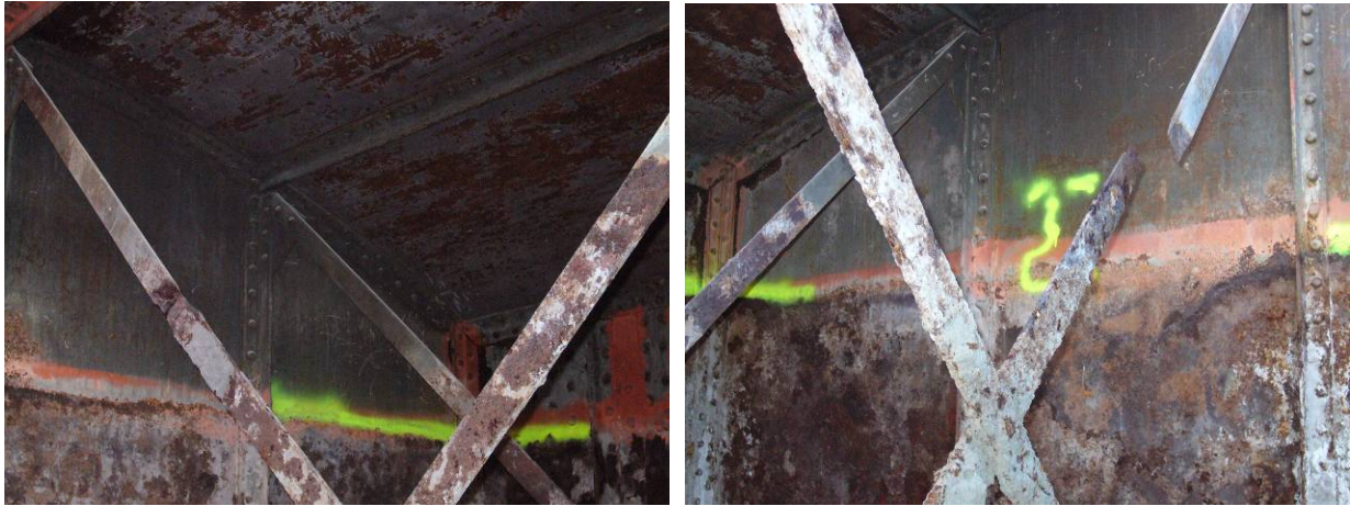
Fig. 5.7.11: bracing cross with cracks due to excessive tensile stress
