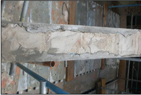
Fig. 4.4.112: Presence of grout in a beam
