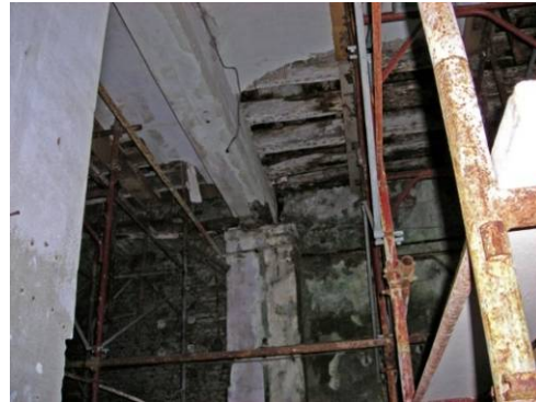
Fig. 4.4.6: Third span: decay of the end beam
