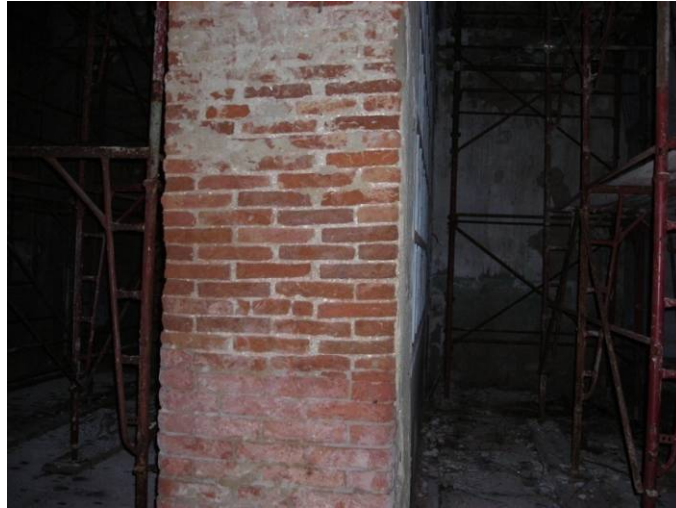
Fig. 4.4.65: Pillar 10 – inclination of the rows of bricks
