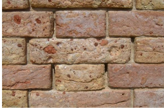
Fig. 5.4.17: ARF's details present in eroded bricks
