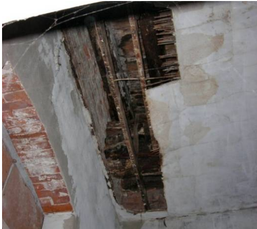
Fig. 4.4.52: Collapse of the false ceiling near the wall
