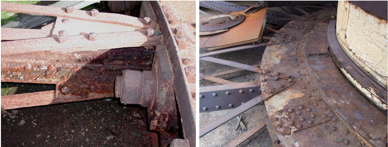
Fig. 5.4.42: slewing ring's corrosion
