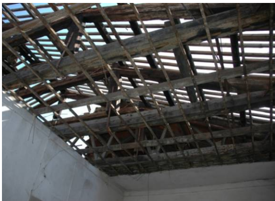
Fig. 4.3.23: System with secondary beam nailed at the tie beam for the anchorage of the false ceiling made with reed wattle
