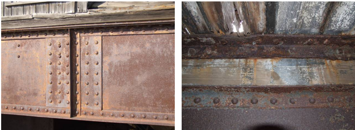
Fig. 5.8.19: Detail of unrecoverable wooden beams
