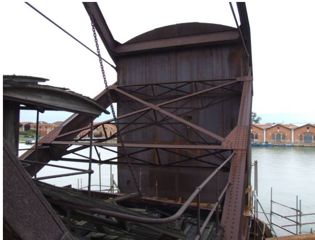
Fig. 5.7.4: Counterweight of the crane
