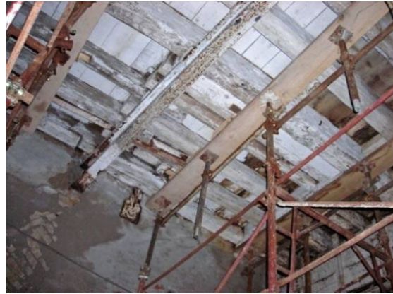
Fig. 4.4.14: End of the beam restrained at the west wall in the walled-up pointed arch
