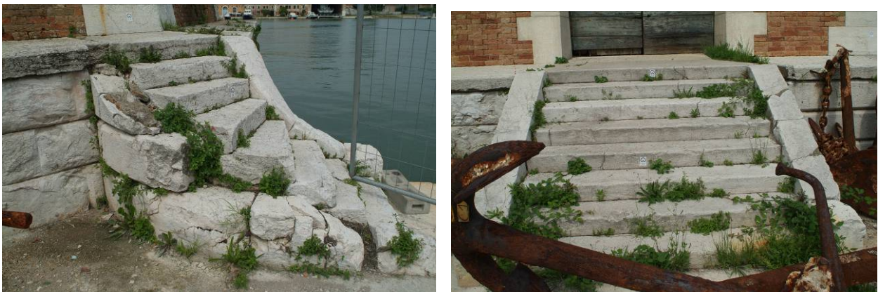
Fig. 5.4.32: The two side stairs with disconnected blocks and missing parts
