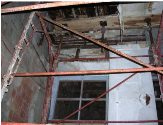
Fig. 4.4.9: Detail of the degradation of the end beam
