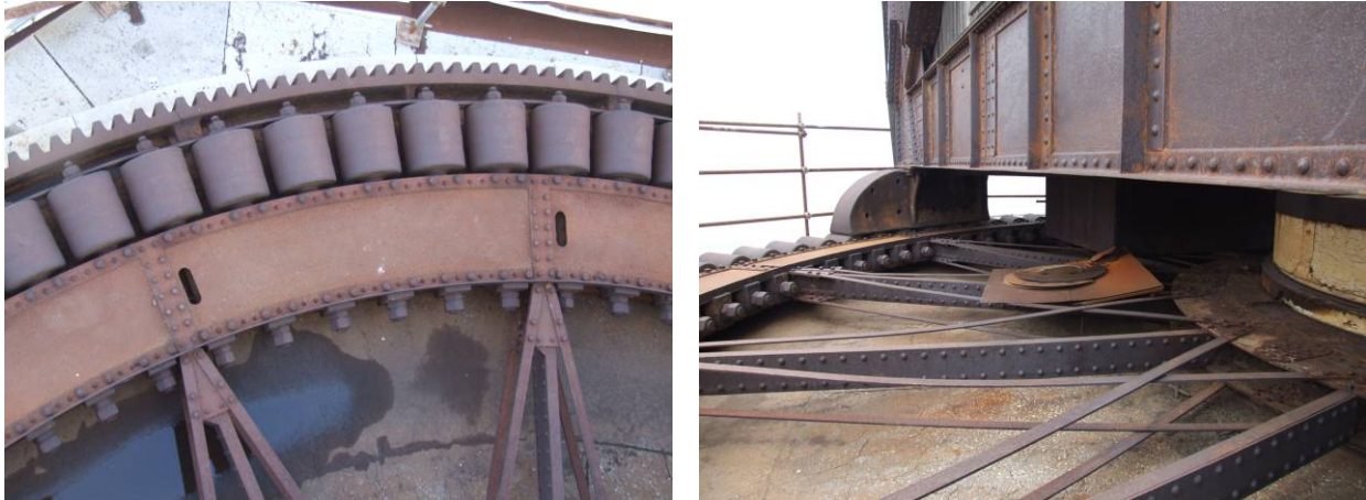
Fig. 5.8.28: Backwater problems at the top of the vault
