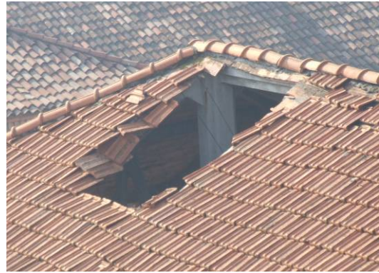
Fig. 4.4.118: View of the pillar of the truss through a hole in the surface roof
