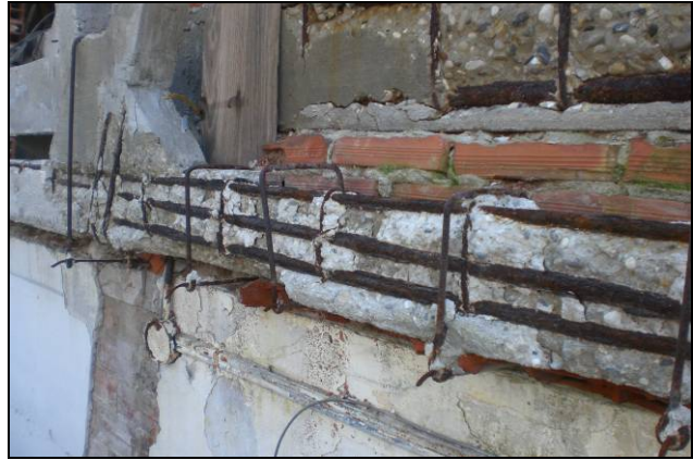
Fig. 4.4.107: Detail of the spalling phenomenon in the tie beam of the r.c. truss of the area B
