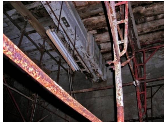
Fig. 4.4.12: Strengthening of one end of the beam through the application of side wooden planks connected to the original beams through metallic rods
