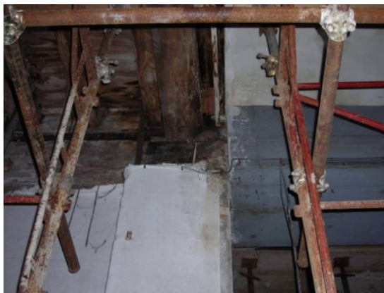
Fig. 4.4.66: Pillar 12 – absence of the slab of stone for the connection beam-wall
