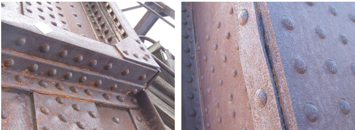
Fig. 5.8.17: Separation between the cracks of the profiles
