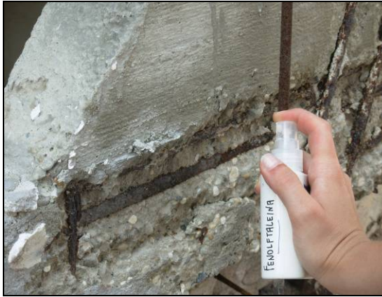
Fig. 4.4.106: Detail of the carbonation phenomenon in a joint of the r.c. truss of the area B
