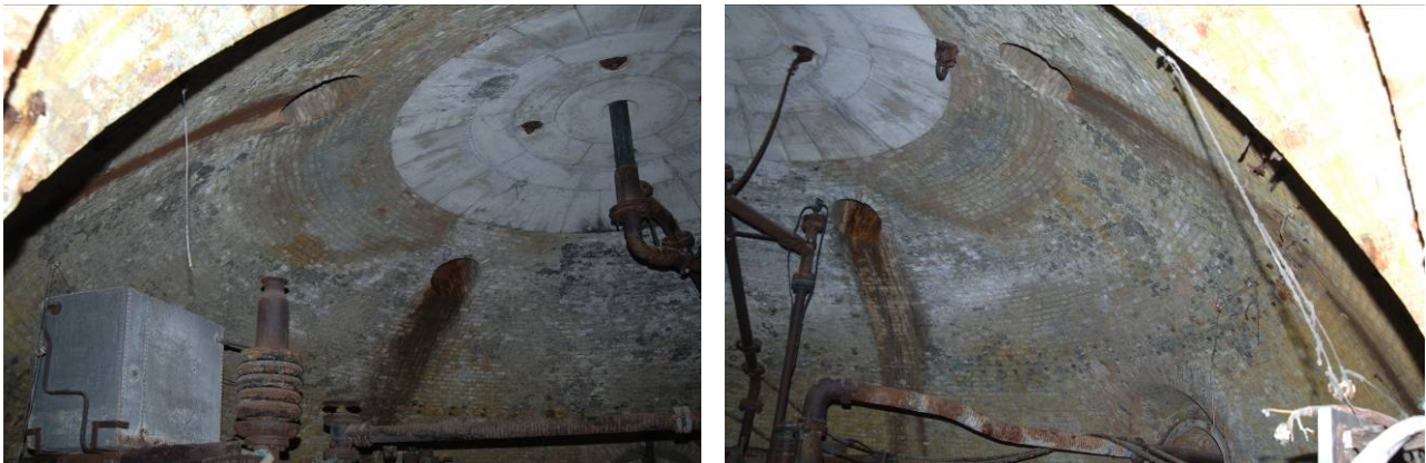
Fig. 5.4.34: Internal surface of the vault showing the light spots covered by efflorescence and the dark ones covered by oxides.
