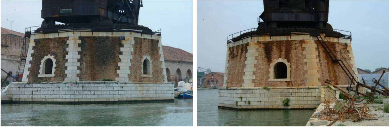
Fig. 5.4.24: On the left the north east side of the basement, on the right the south west side of the basement
