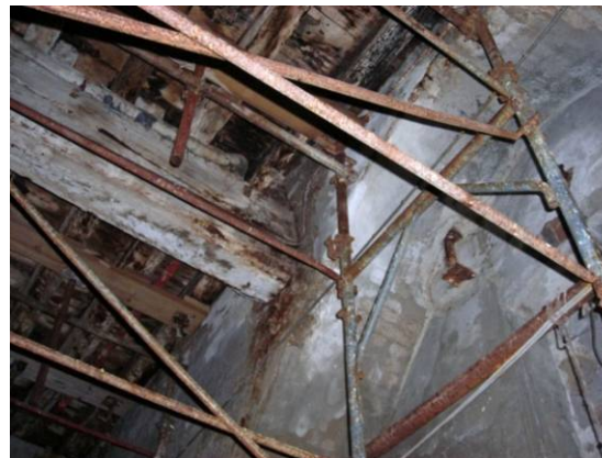
Fig. 4.4.10: The end of the beam located near the pointed arch of the west wall
