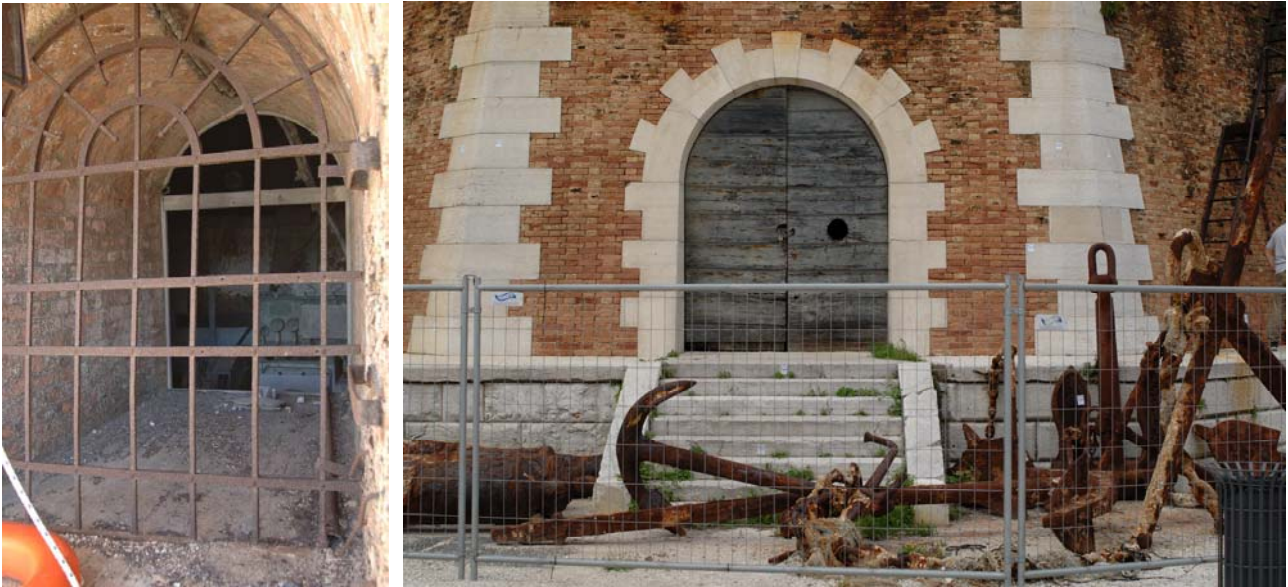
Fig. 5.8.25: Details of the windows and of the wooden door of the basement
