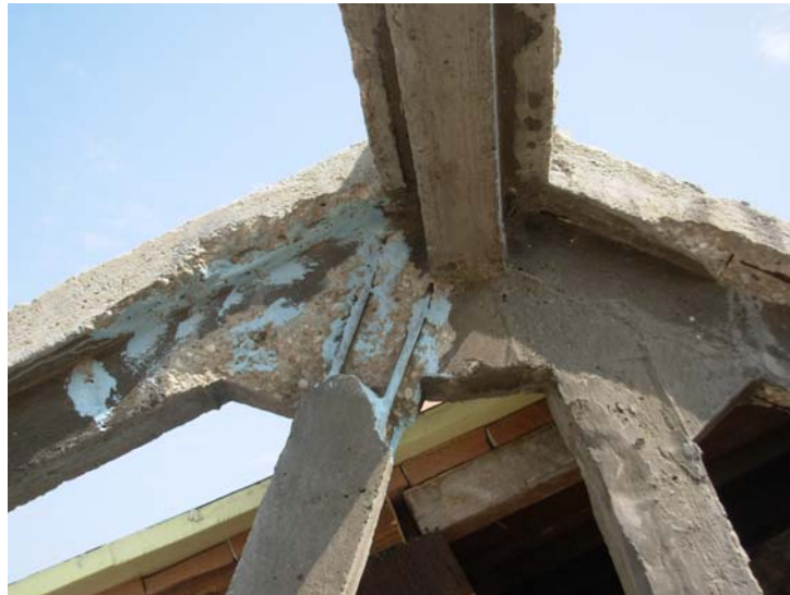
Fig. 4.6.34: Detail of the decay of the joint struts-secondary elements
