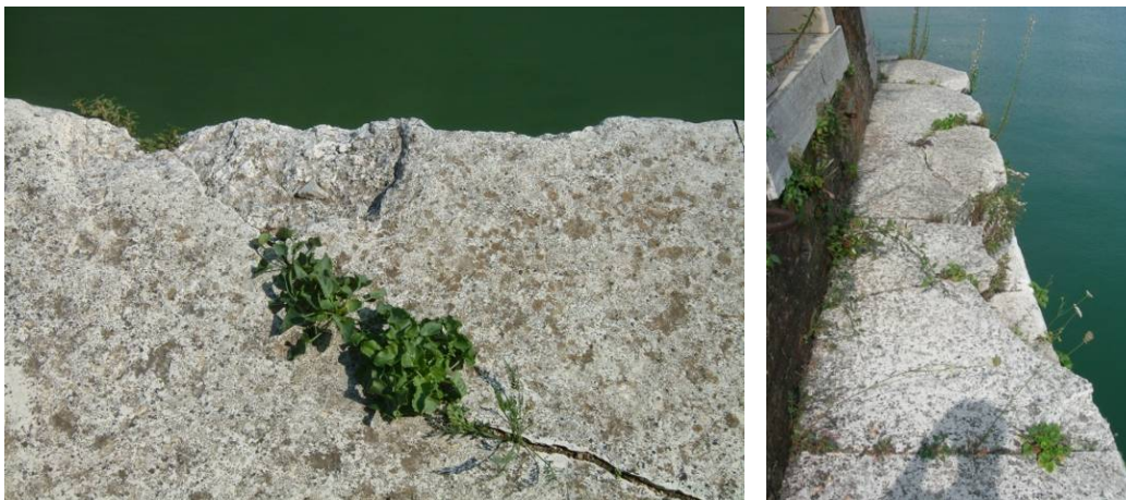
Fig. 5.4.31: Degradation cause by biological patina
