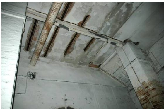
Fig. 4.3.21: Floor features by hollow tile placed in the flanges of the iron beams
