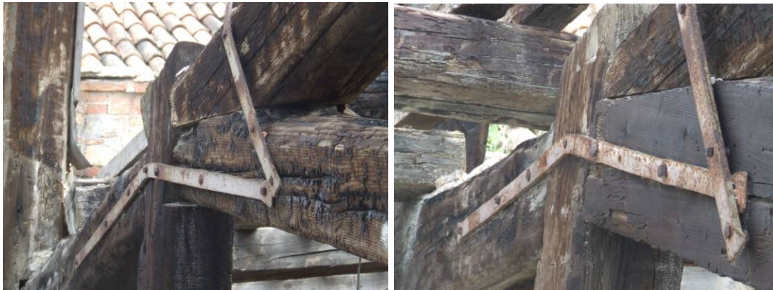
Fig. 4.4.81: Degradation of joints
