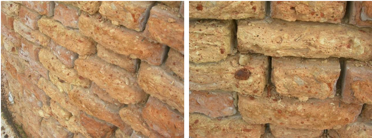
Fig. 5.4.25: Eroded surface's detail
