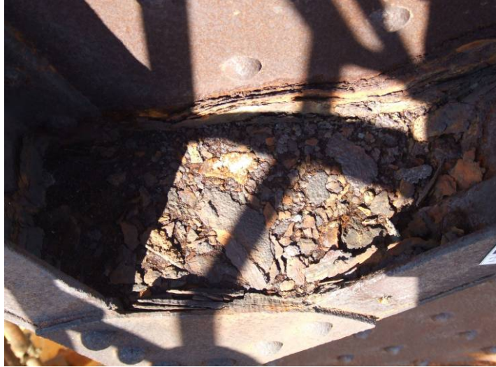
Fig. 5.4.41: Drainage of the main ruster, blocked by the corrosion products.
