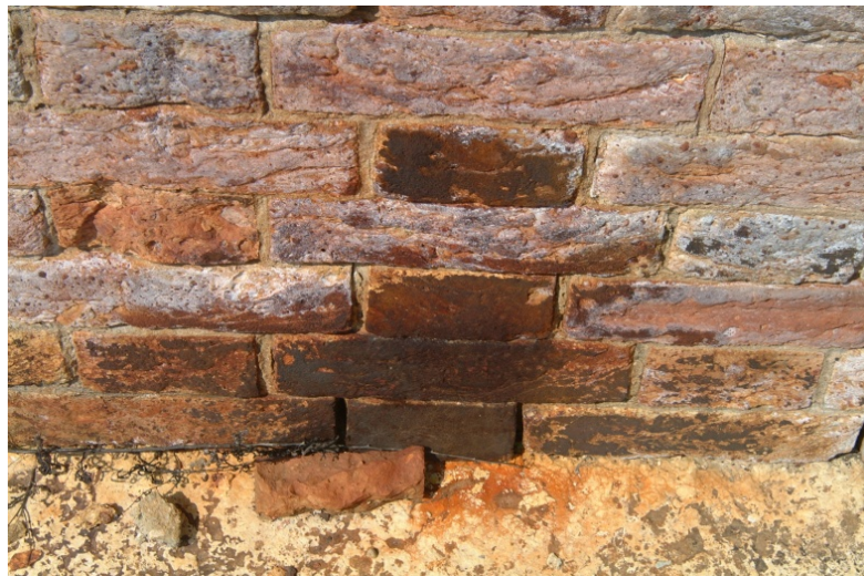
Fig. 5.4.27: Corrosive deposits stains
