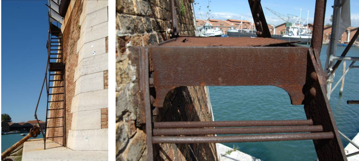
Fig. 5.8.18: Stairs and landings degradation
