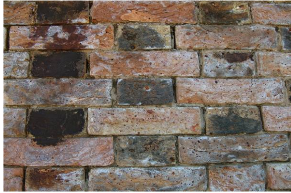
Fig. 5.4.26: Masonry's detail showing that efflorescence is not present on the surfaces covered by corrosion's products and dark stains
