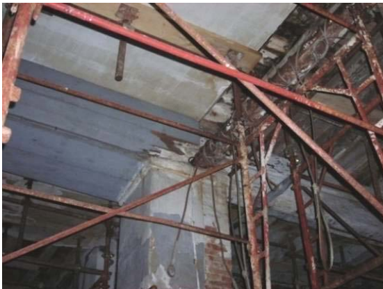
Fig. 4.4.11: Wooden coating in the first span; support the beam on the pillar 12
