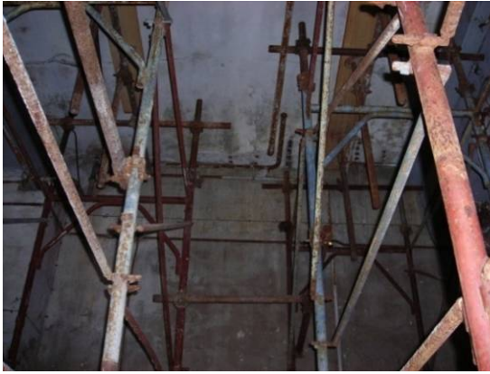
Fig. 4.4.28: View of the false ceiling where it is possible to see the metallic net
