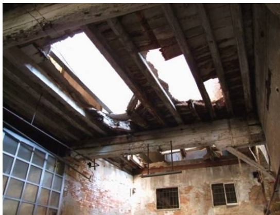
Fig. 4.4.54: Partial collapse of the floor
