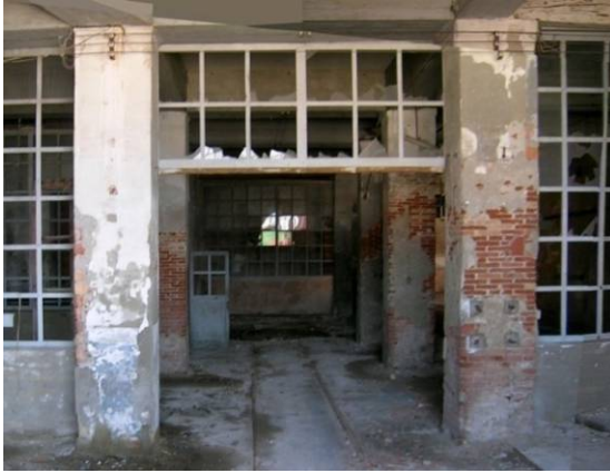
Fig. 4.4.63: Pillars 6 and 7 with diffuse detachments of plaster
