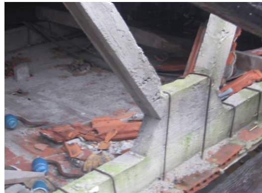
Fig. 4.4.109: Detail of a poor concrete in a joint
