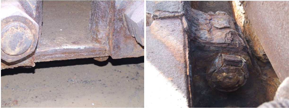
Fig. 5.8.13: Details of the metal elements degradation
