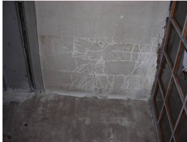
Fig. 4.4.53: Effects of the moisture rise in the false ceiling plastered
