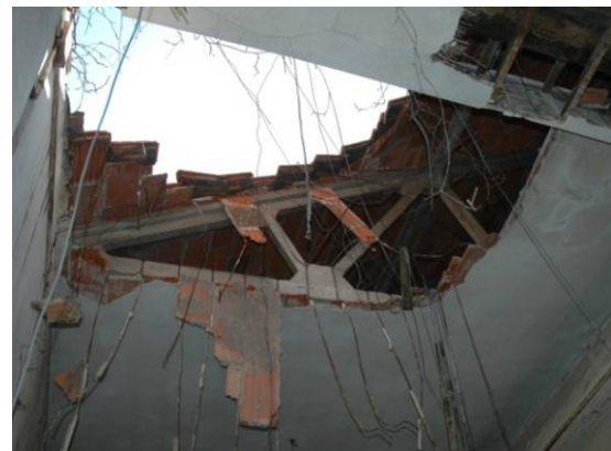
Fig. 4.3.24: Collapse of the "Perret" false ceiling, anchored at the reinforced concrete truss, as a consequence of the collapse of the tile roof
