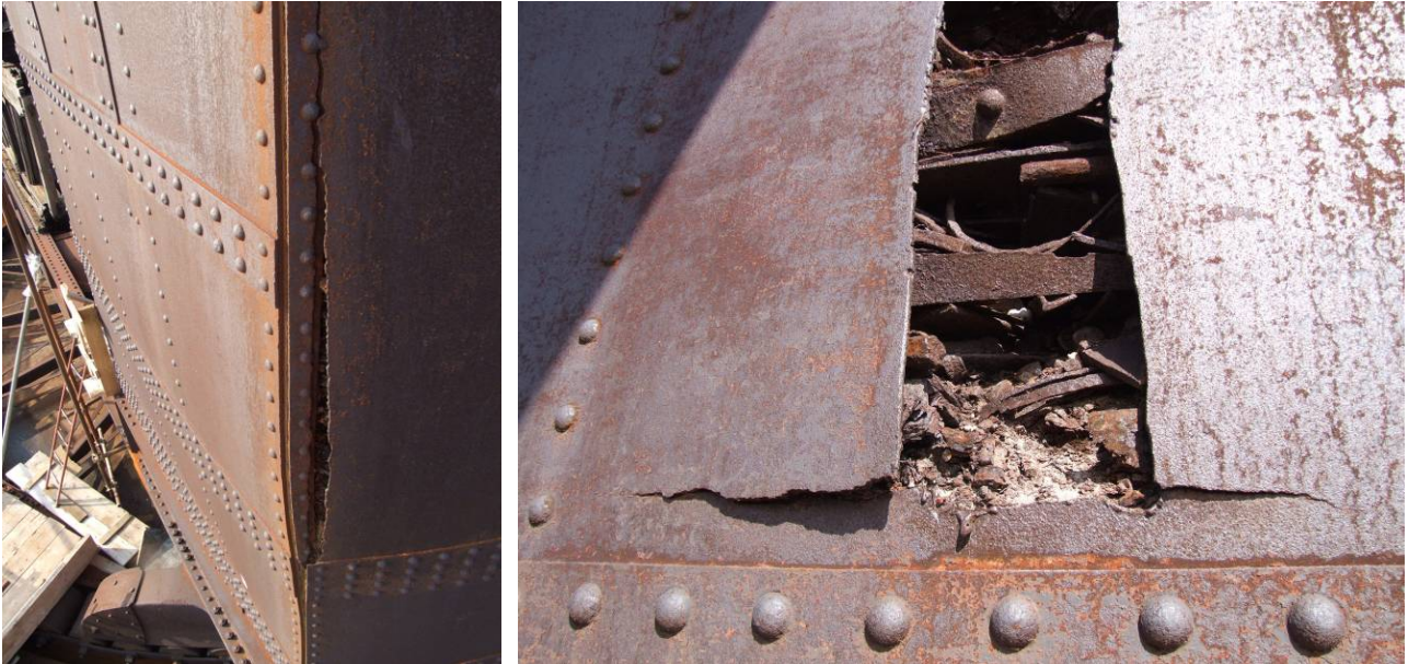
Fig. 5.4.51: Crack on the rear of the counterweight and in particular on one of the inspection holes present in the box
