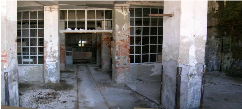
Fig. 4.3.12: Ground floor entrance on the north side: room characterized by two rows of pillars
