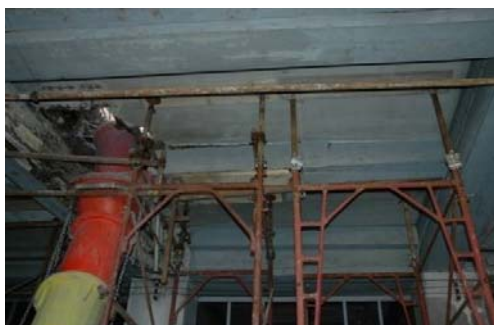
Fig. 4.4.30: Collapse of the floor
