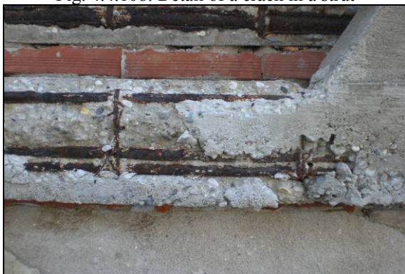
Fig. 4.4.110: Detail of concrete swelling in a tie beam
