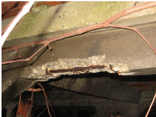
Fig. 4.4.108: Detail of a crack in a strut
