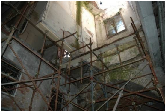
Fig. 4.4.56: Total collapse of the floor
