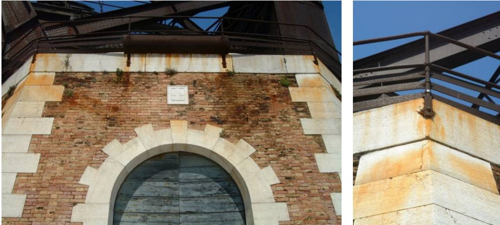
Fig. 5.4.33: Corrosion deposits stains on Istria stone
