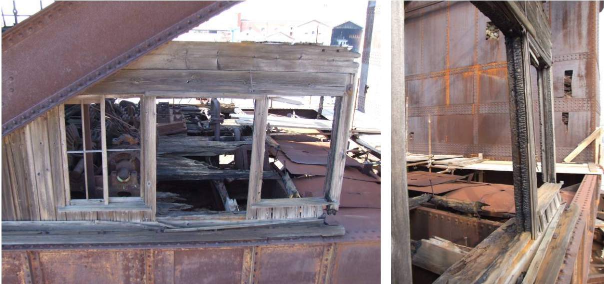
Fig. 5.8.20: Conditions of the cabin after the fire
