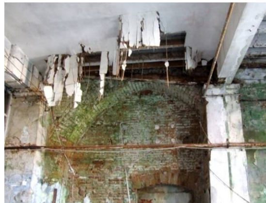
Fig. 4.4.33: Collapse of the support of the edge beam
