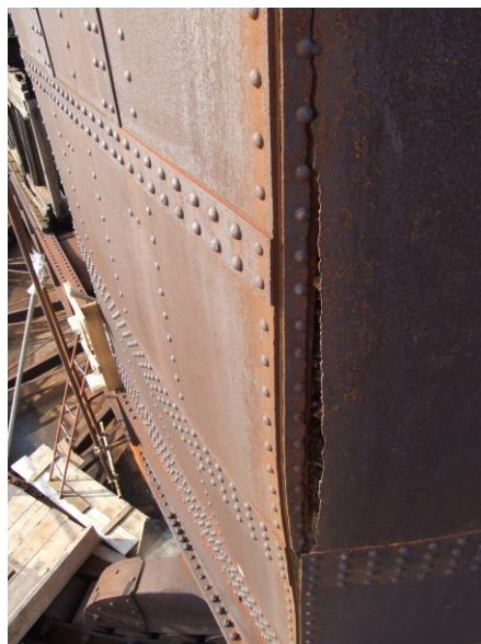
Fig. 5.7.6: Crack in the north elevation of the caisson
