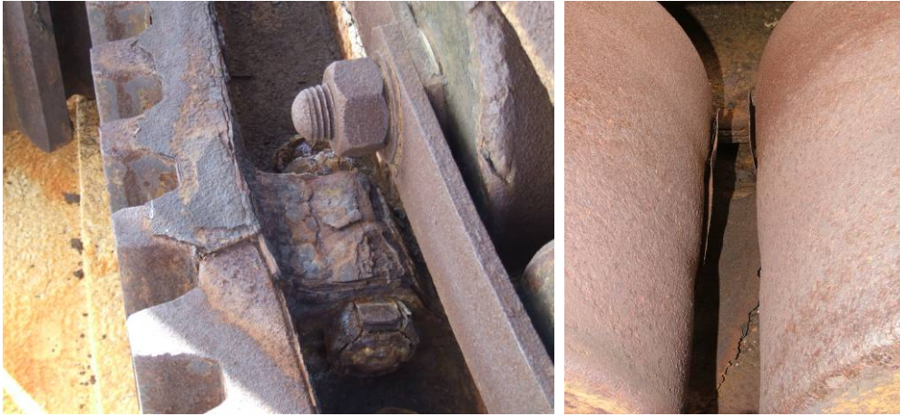
Fig. 5.4.46: Rack's corrosion and rollers exfoliation
