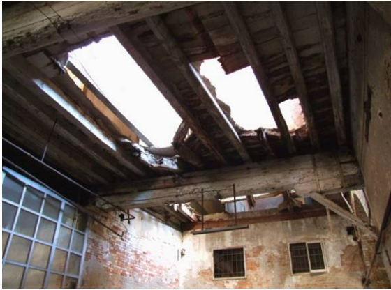
Fig. 4.3.19: A venetian traditional flooring emerged from the collapse of the wooden floor
