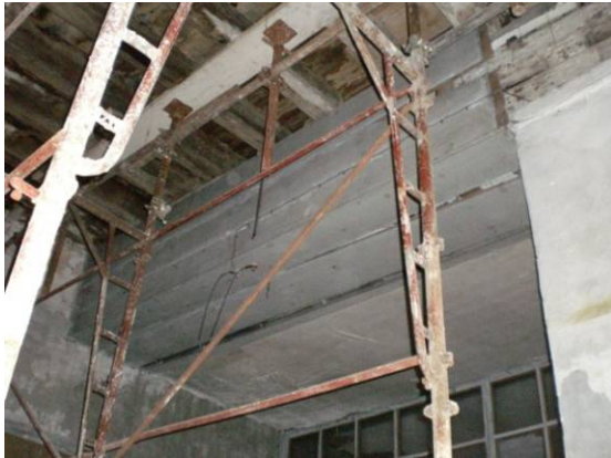
Fig. 4.4.15: Coating in wooden plank for all the span width of the first span
