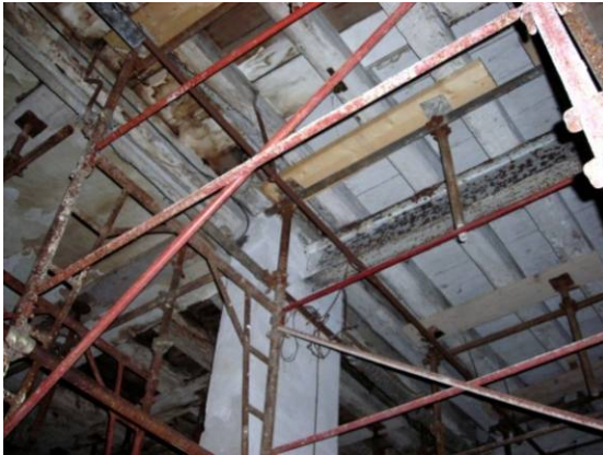
Fig. 4.4.13: The end of the beam restrained at the pillar 14
