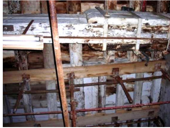
Fig. 4.4.48: Supporting wooden beam to unload the weight of the end of the main beam 4
