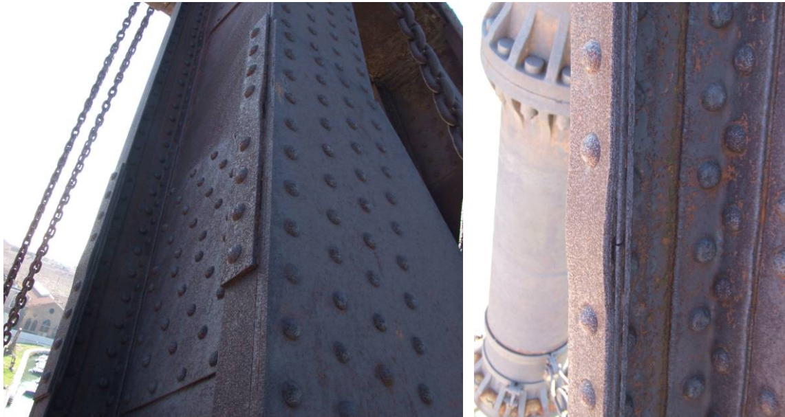
Fig. 5.4.38: Evident open cracks where the rivet pitch is wider and where there are joints.
