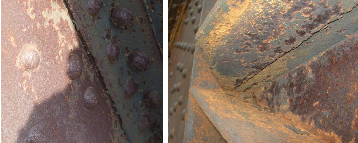
Fig. 5.4.39: The protective layer placed on the surfaces and not yet present on some small areas
