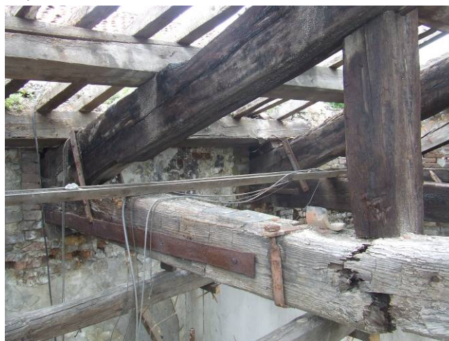
Fig. 4.4.79: Detail of a breaking in the tie beam near the joint with the post
