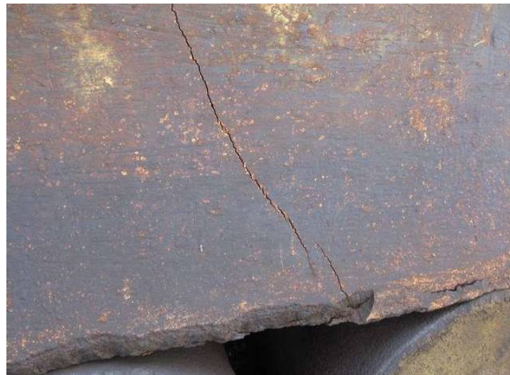
Fig. 5.4.50: Crack on the sliding block below the counterweight
