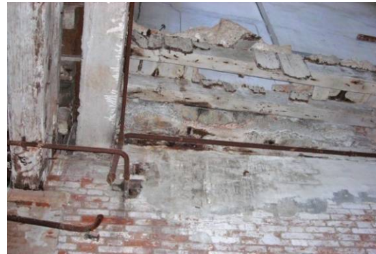
Fig. 4.4.57: Materials decay of the frame
