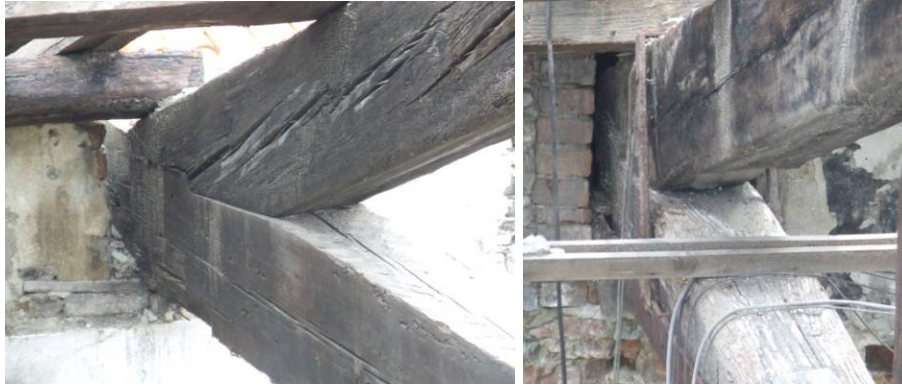
Fig. 4.4.80: Degradation at the ends of beams, near the anchorage
