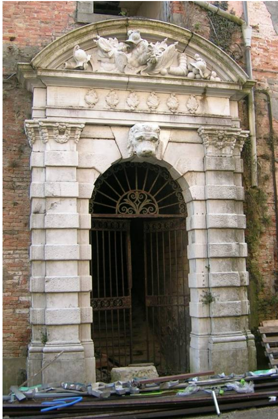
Fig. 4.2.5: Baroque portal at the entrance of the southern “Sale d’Armi” on the “Stradal Campagna”
