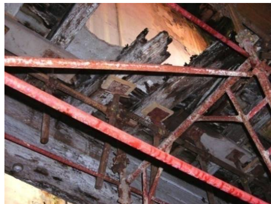
Fig. 4.4.55: Purlins and plank collapsed as a result of the material decay
