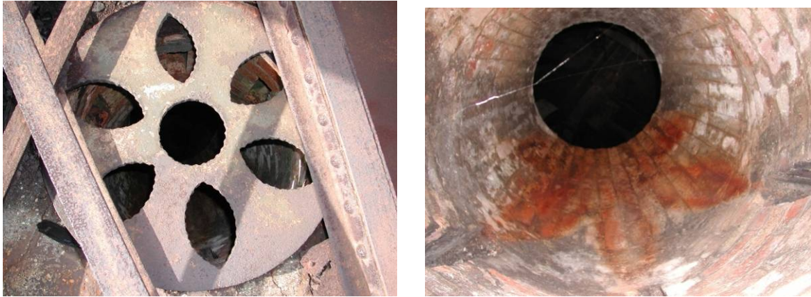
Fig. 5.4.35: The basement's holes from which the superficial whasing products enter
