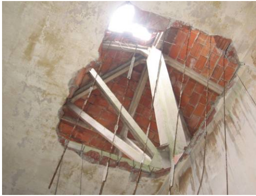
Fig. 4.4.117: View of the trusses and of the pillar through a hole in the false ceiling
