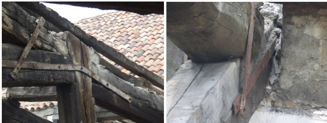
Fig. 4.4.82: Degradation of joints and of the connection between masonry wall and tie beam
