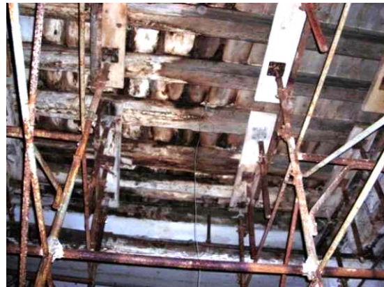
Fig. 4.4.39: Purlins and plank moisture
