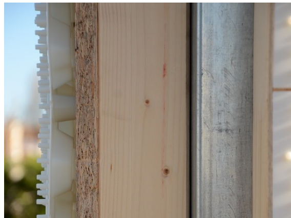
Fig. 4.12 – Wall section: (from left to right) skin, OSB panel, timber stud, steel column.
