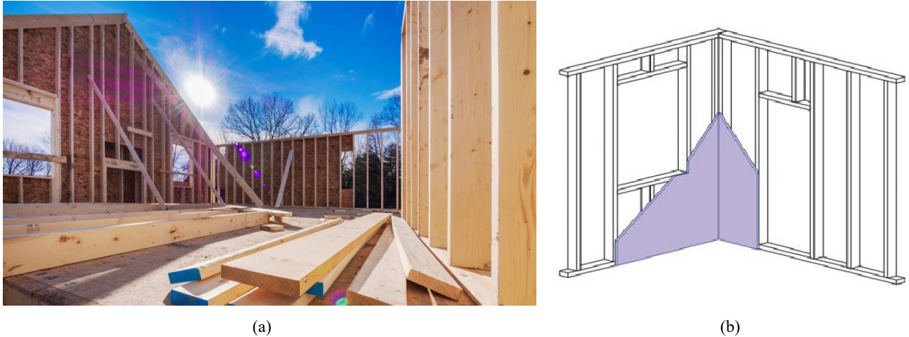
Fig. 1.6 – Platform-frame system. (a) Example of building [I.18]; (b) bracing of light frame [I.19].
