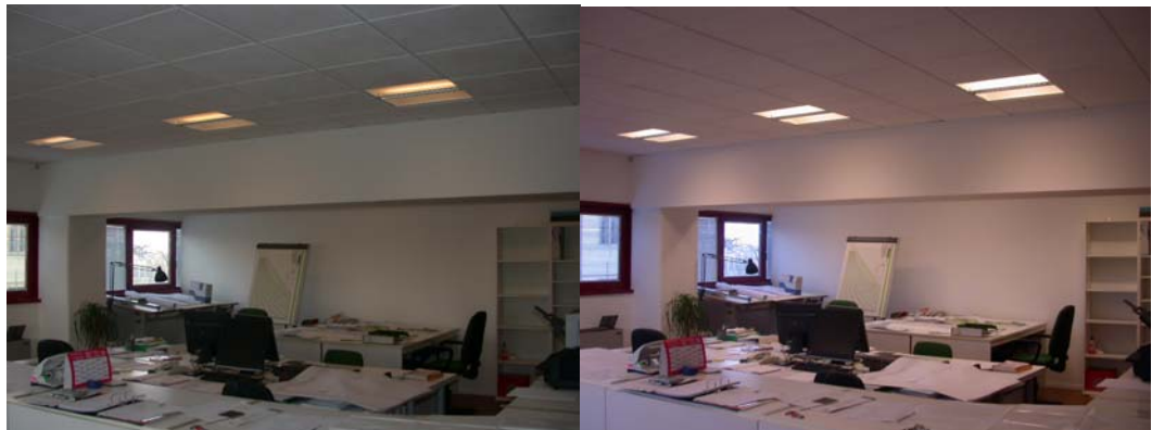
Figure 8-102 The lighting system without daylight control (left) and with day light control (right)
