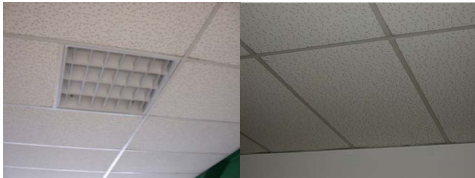
Figure 8-94 Old luminaires and old plaster ceiling
