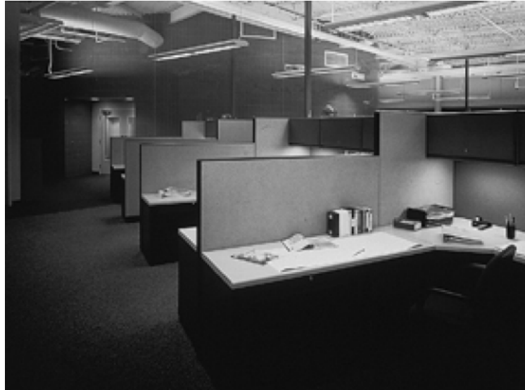
Figure 7-13 An open-plan office with direct-indirect fluorescent luminaires in a regular pattern, providing ambient light for the workstations beneath.
