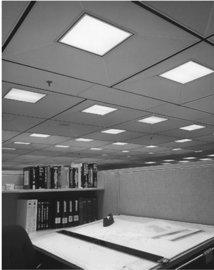
Figure 7-10 Direct lighting from a fluorescent system that provides good general illumination as well as adequate light for working at the drafting table.
