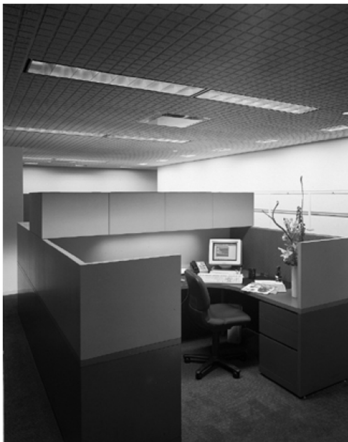
Figure 7-7. A workstation with built-in task lighting illuminating the desk top below. The low brightness ceiling luminaire with parabolic louvers cuts down on reflections on the VDT screen.
