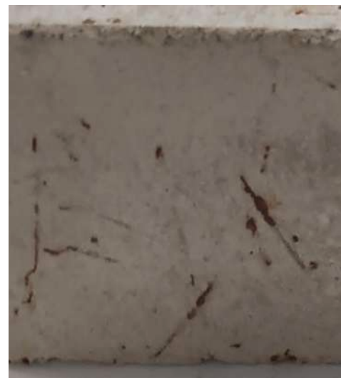
Fig. 17. Detail of the corrosion of external metallic fibers after the SO 2 -attack test on a mix SC/II-M specimen.
