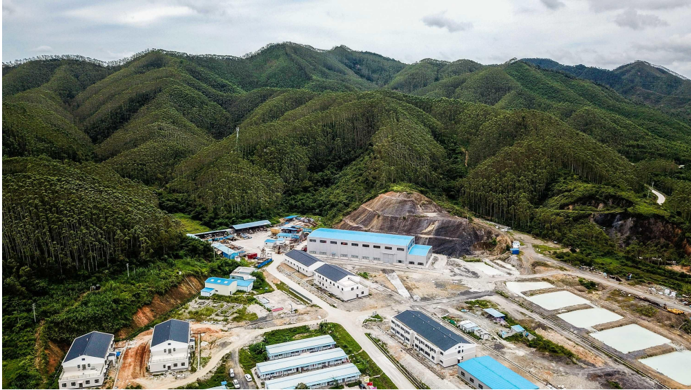
Figure 3.2: Aerial photograph taken on June 23, 2019, showing the construction site of JUNO. Taken from [52].
