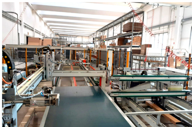
Figure 6. Part of the newly installed packaging line (Case 1—own research).
